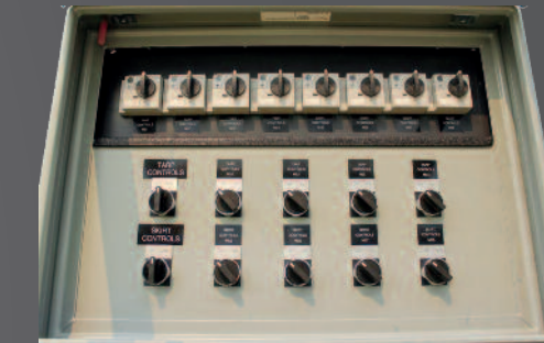
CONTROL PANEL for tarp and skirts
