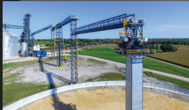
Complete temporary storage systems consisting of center air tower, conveyor trusses, support towers, Material handling, tarp and aeration tubing
